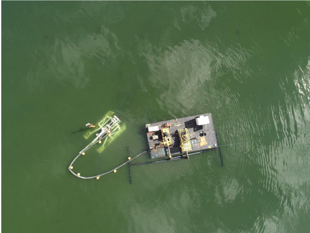
Figure E-1. Stationary jet plow in position with pump barge, prior to start of jet plow. 11:52 AM, Sept 9, 2019.
